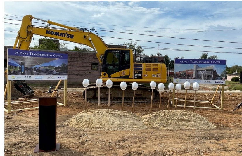
On October 4 th , 2021, Albany Transit System broke ground on a new downtown multimodal transit facility at 300 West Oglethorpe Blvd.
